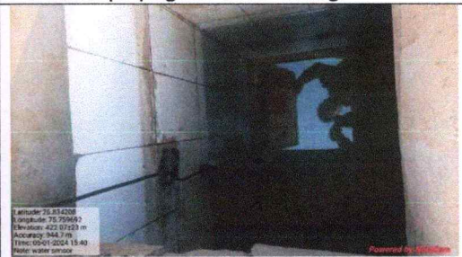
P4: Water sensor in the tank.
