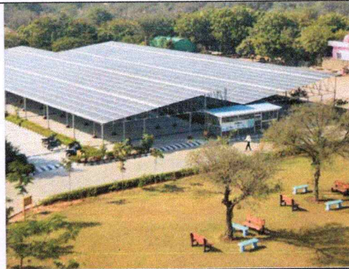
K1: solar panel above the parking area
