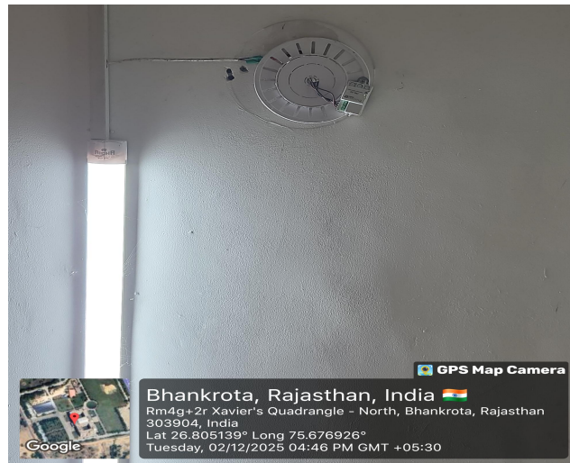
Figure 9: Motion/ Occupancy Sensor
