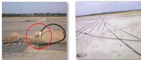
Figure 4: Illegal Borewells and Electric Cables around Sambhar Region
